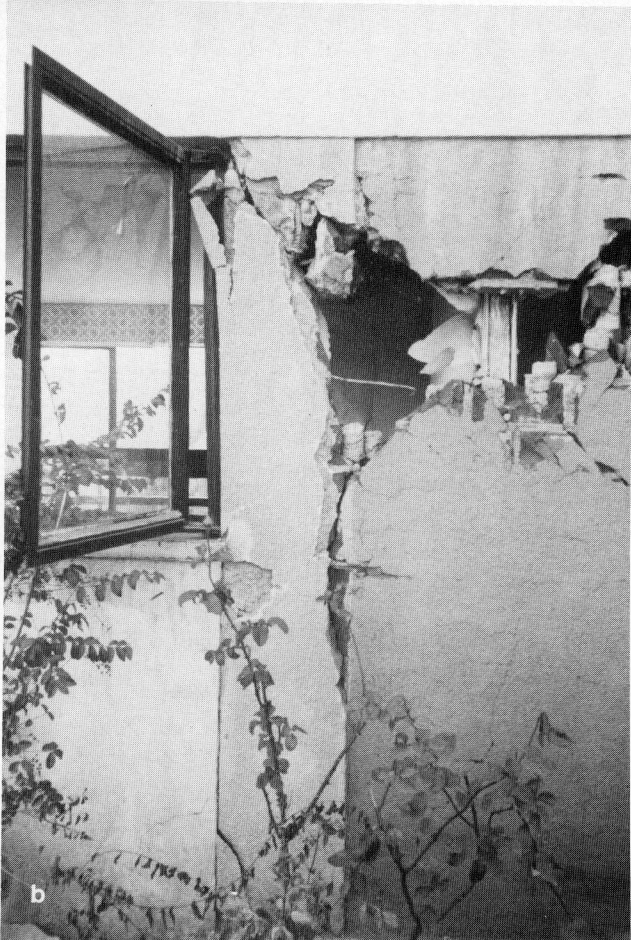
FIG. 7. (a) A typical damaged four-story building on a ridge and (b) close-up of damage to structural components.
