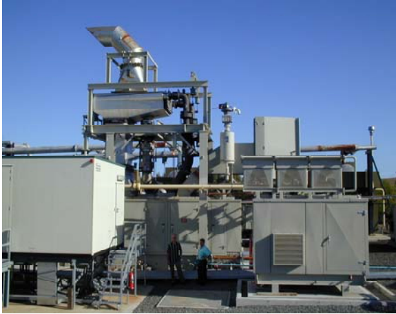
Lean fuel turbine running off of ventilation air methane and drained gas. (Courtesy of Energy Developments Ltd.)
