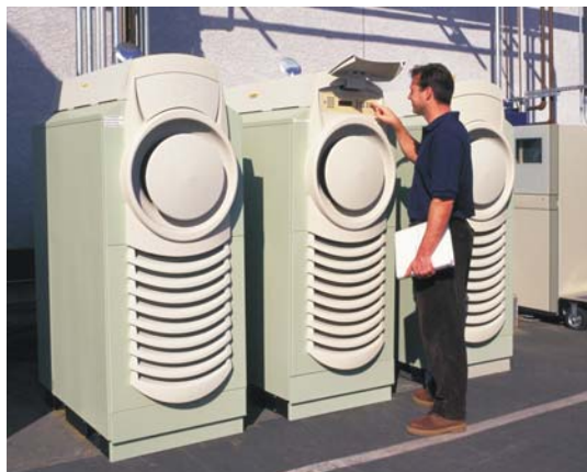
Three 30-kW microturbines are in use at a landfill in Burbank, California, to generate electricity.
