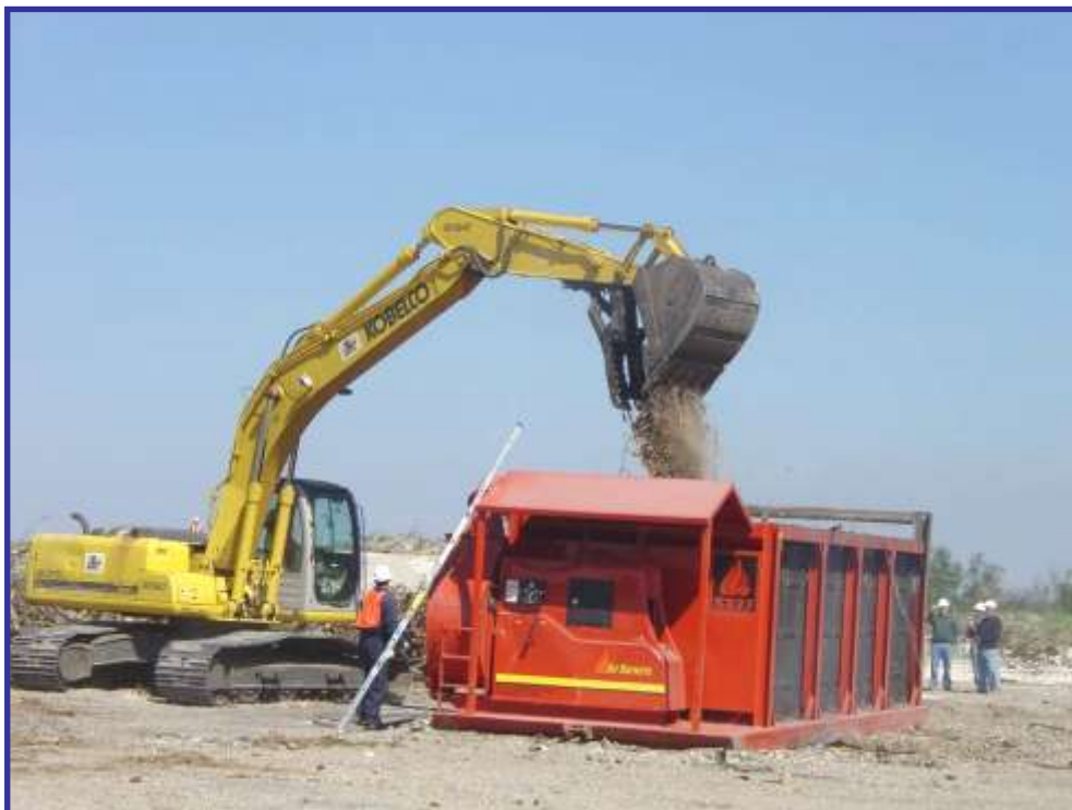
Figure A-2. ABT Unit (Model S-327, Air Burners, LLC) used in Phase I performance evaluation at Amid Landfill in New Orleans, LA (October 24-25, 2005).
