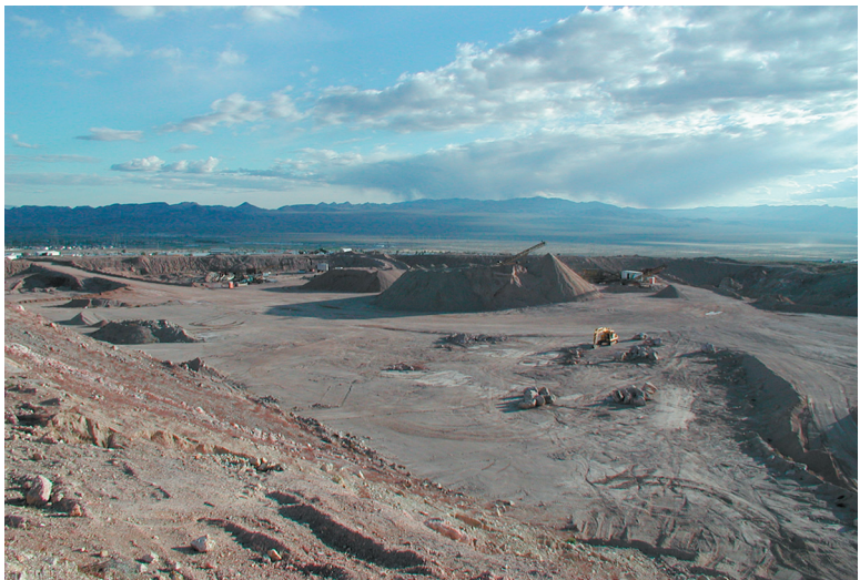
Figure 10. The Bootleg Canyon aggregate pit, a sand and gravel mining operation about 2 km southwest of the River Mountains ACEC.
