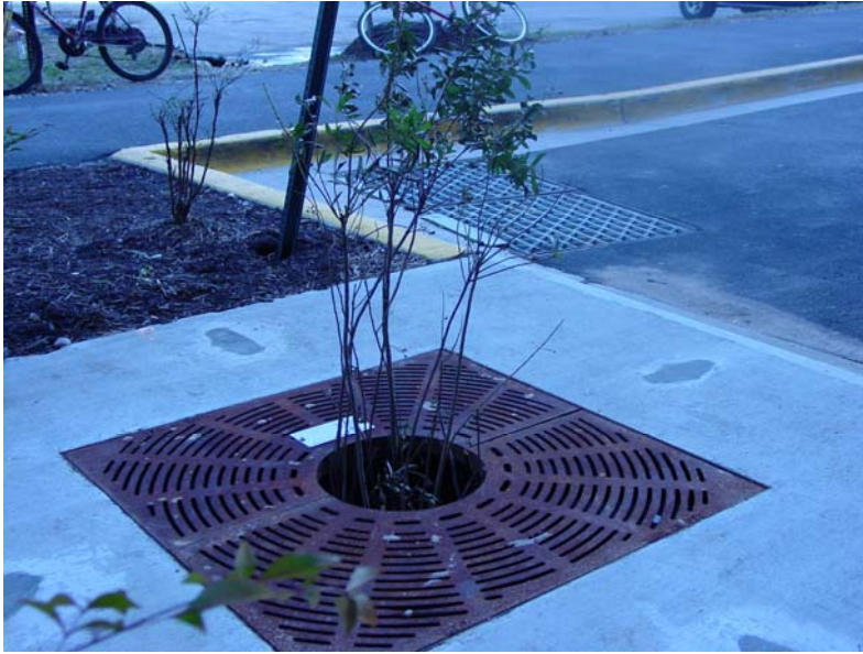
Figure 15: Vegetation used for stormwater management at University View
