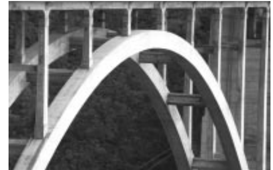
Operating and maintaining infrastructure account for a large share of local government costs.
