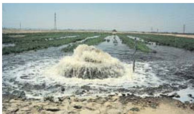
Pumps transfer water from the withdrawal wells to irrigation zones in the Negev Desert, Israel. Photo courtesy of Bahman Sheikh
