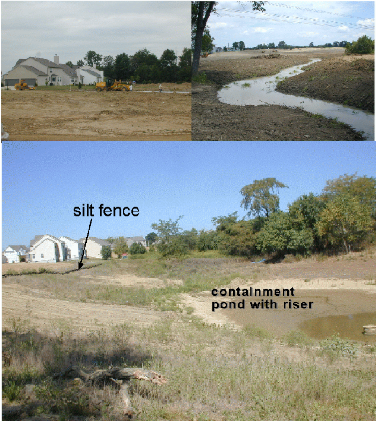
Figure 4. Construction sites observed in the rapidly suburbanizing Columbus, Ohio metropolitan area. Upper left, a construction site in the Rocky Fork watershed; the exposed soil is supposed to be stabilized with straw and seeded with grass. Upper right, another tributary bulldozed for new construction. Lower picture, a construction site in Fairfield County instituting proper environmental controls including silt fencing and a settling pond.
