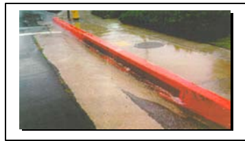
Figure 14. Catch basin screen operating during storm. Water can flow through the openings while keeping trash out.
