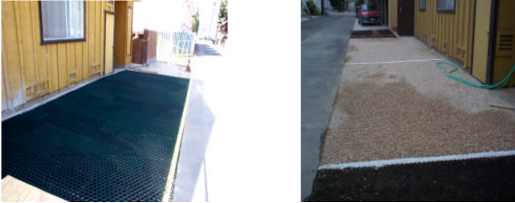
Figures 9, 10. On left and right, before and after photos of Grassy Pavers permeable pavers at a multi-family building in the parking stalls. Left photo shows pavers exposed before infill. Right photo shows pavers filled with colored rock.
