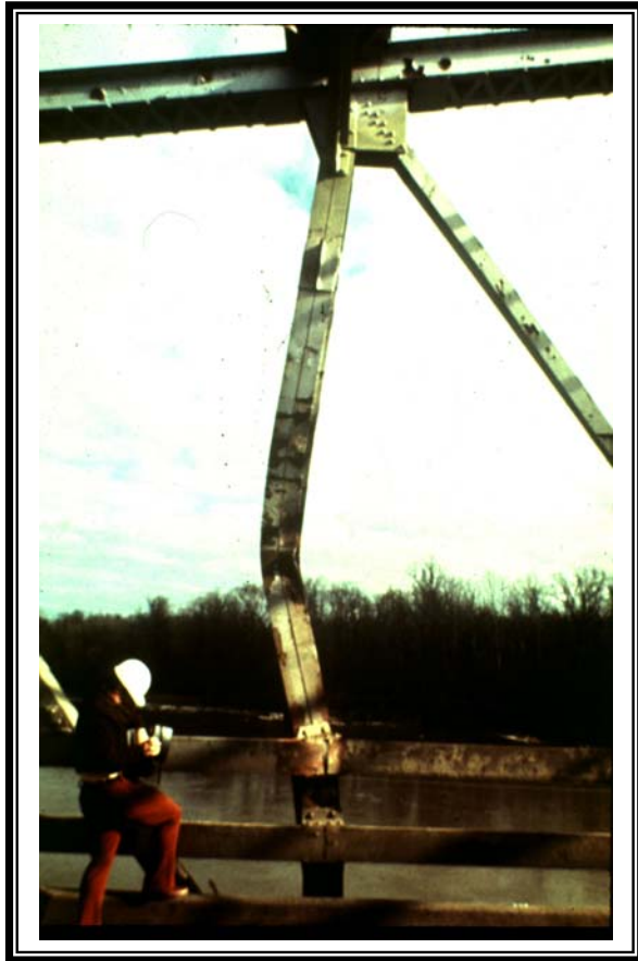
(a) Category W damage on a built-up double channel truss member. The damage was caused by a log falling from a truck on a bridge in North Louisiana.
