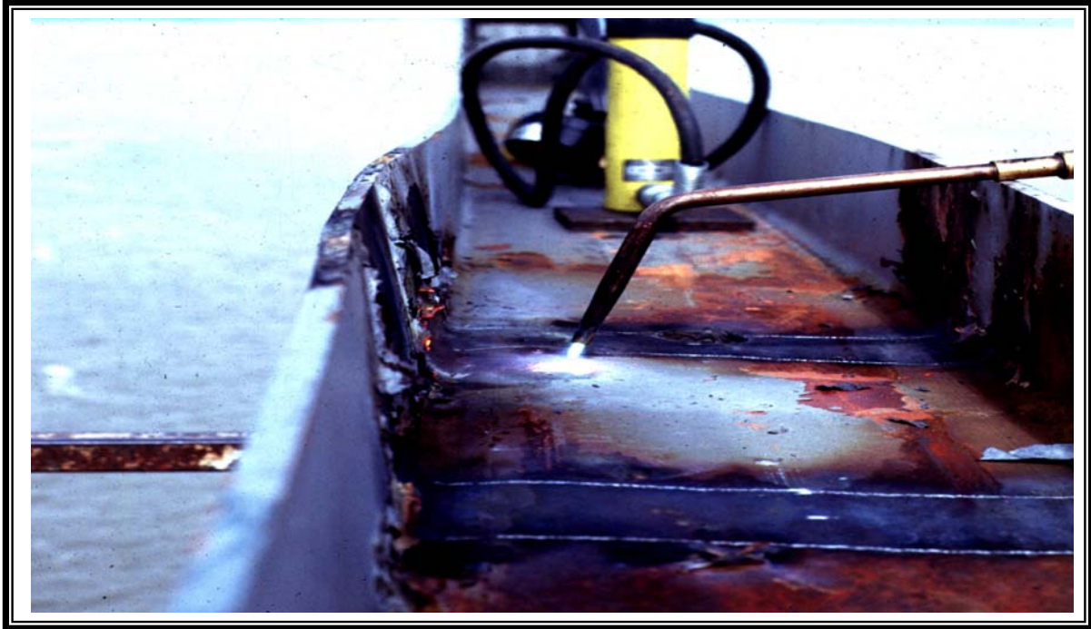
Figure 10. Strip heat in progress with a completed strip heat in the foreground.
