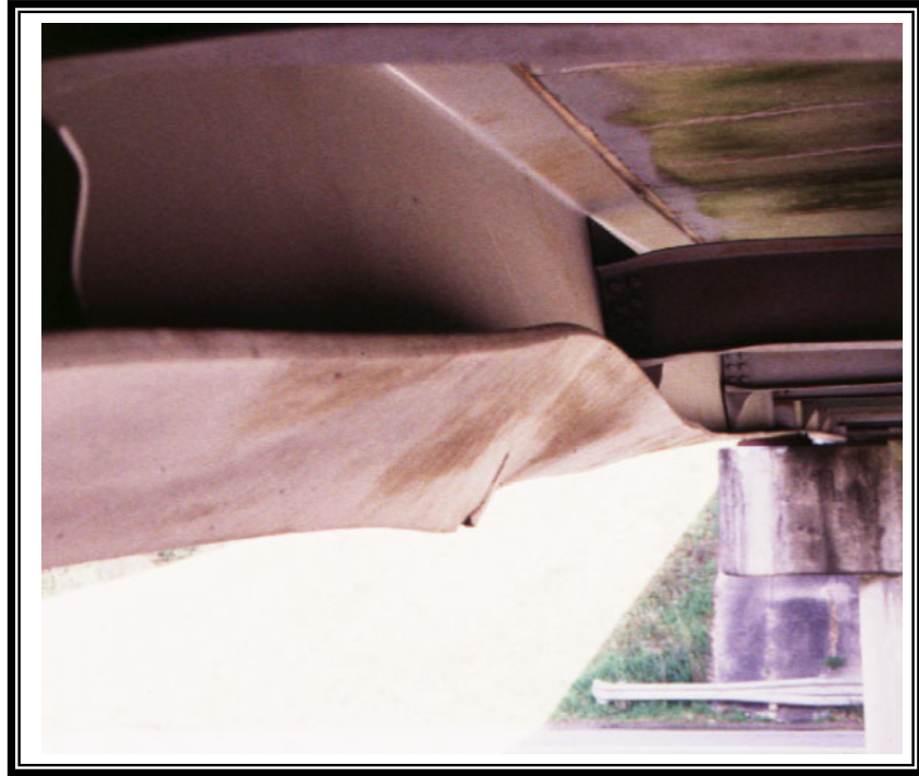
Figure 24. Diaphragm damage due to vehicle impact on girder.
