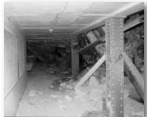
The damaged Cortlandt Street subway station, just east of the World Trade Center. This stretch of track will be closed for years because the ceiling of the tunnel caved in beneath the rubble of the collapse.
