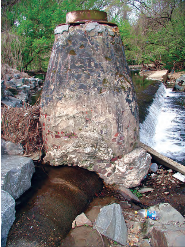
Figure 27. Exposed sewer manhole stacks in Sligo Creek, a small tributary on the Northwest Branch Anacostia River. (Photograph courtesy of the Anacostia Watershed Society.)
