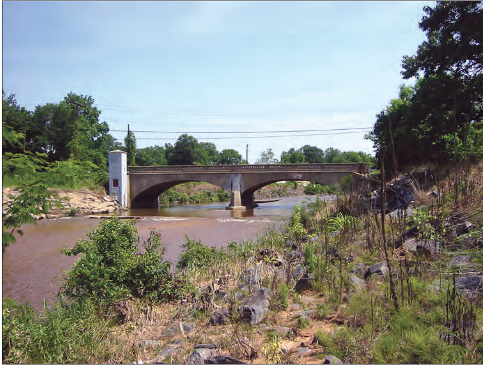
Figure 2. The historical stream gage (at left end of bridge) at the Northeast Branch Anacostia River at Riverdale, Maryland (USGS station 01649500). (Photograph by U.S. Geological Survey)
