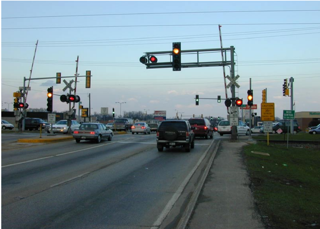
Figure 50. Pre-Signal Mounted on Railroad Cantilever, Rollins Road and State Route 83 at Wisconsin Central, Round Lake, Illinois
