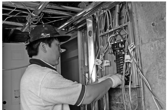
Electricians may rewire a home and replace an old fuse box with a new circuit breaker box to accommodate additional appliances.
