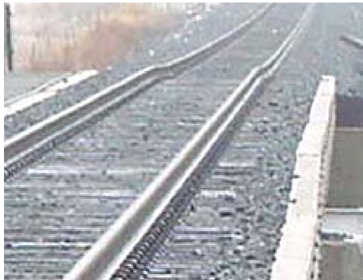
Figure 1. Track settlement off a bridge end
