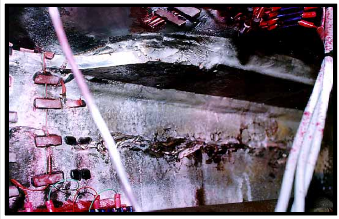
Figure 12. B-End Right Corner Flaw and Tank Head Rosette
