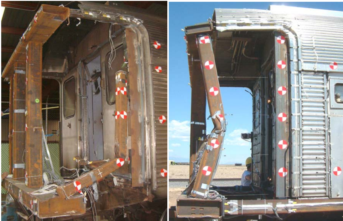
Figure 9. Photographs Comparing the Corner Post Crush of the 1990s (Left) and SOA (Right) End Frame Designs
