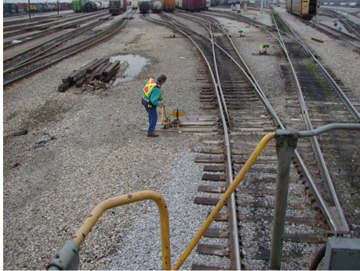
Figure 7. RCO lining switch
