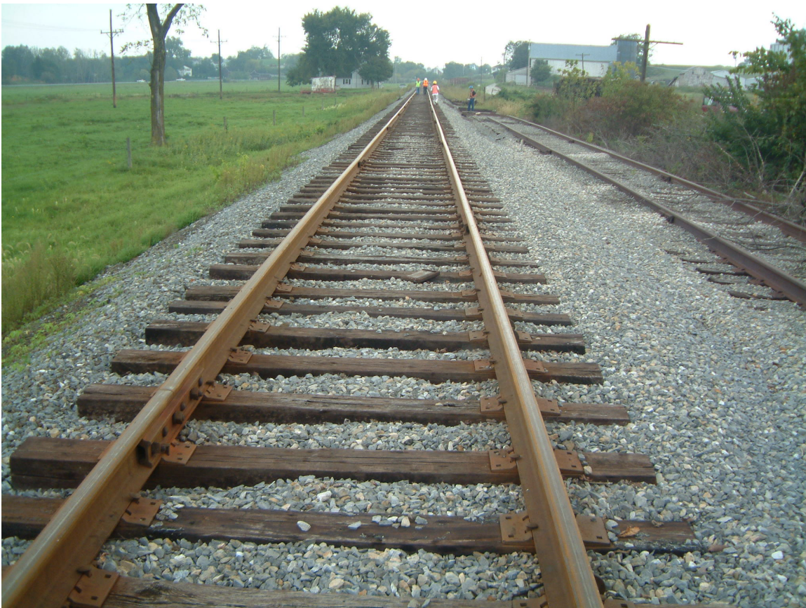
Figure 3. Tangent Track Section East of Union Bridge Used for Phase II Testing
