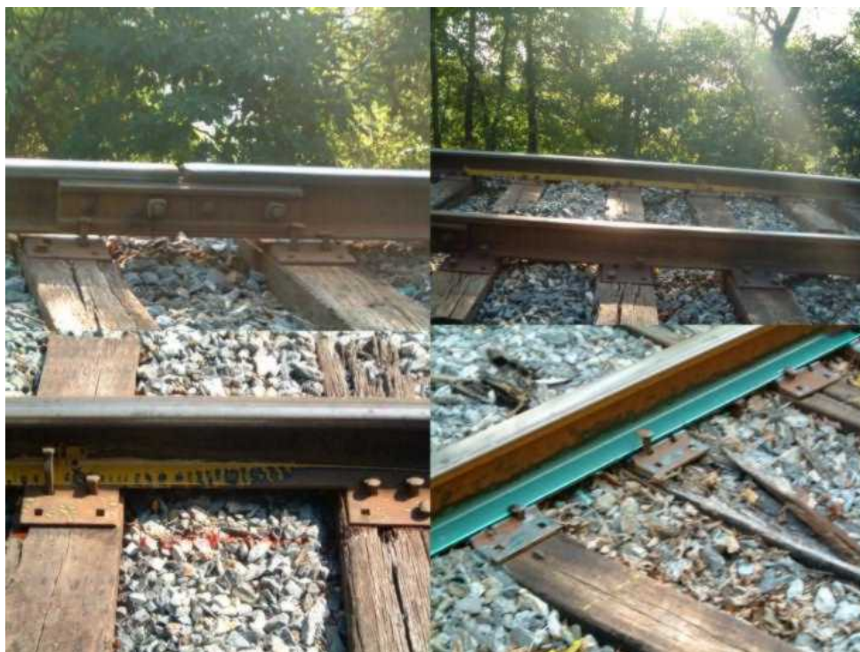
Figure 2. Typical Track Sections Where Both Test Vehicles Detected Defects
