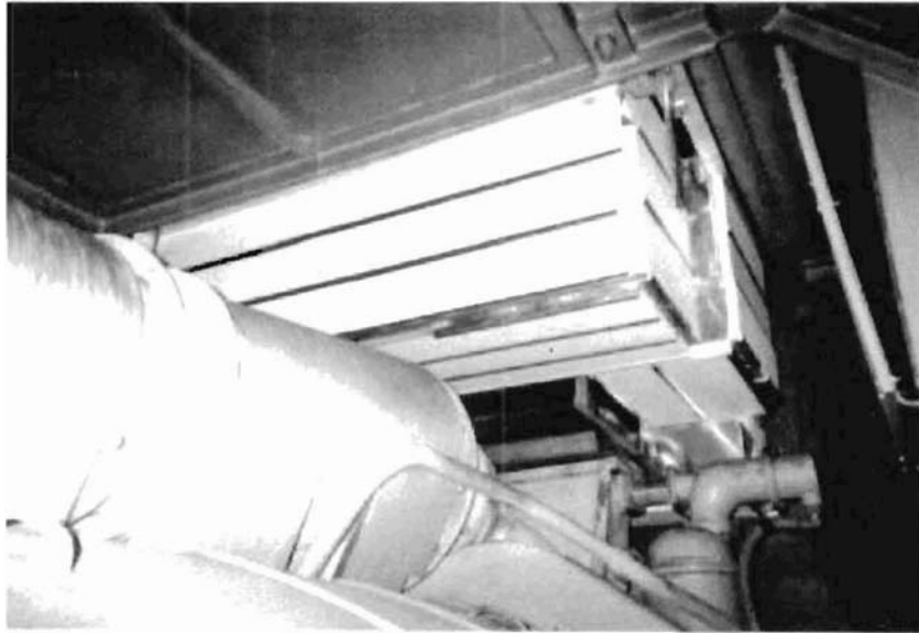
Figure 79. The Cool Box Installed in the Locomotive
