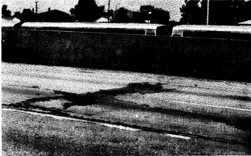
c. Pavement in poor condition. About 9 percent of all Interstate highway mileage was in this condition in 1978. Poor pavement is in extremely deteriorated condition, and may need new sub-base and base material in addition to resurfacing. The above section exhibits high-severity longitudinal cracking in the center lane.
