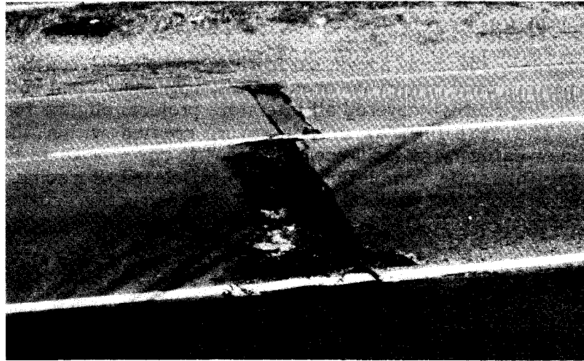
d. Pavement in poor condition. Same characteristics as photograph c. The above section shows high-severity joint load transfer system associated deterioration.
