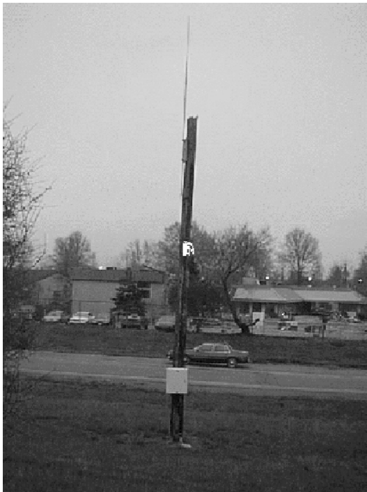
Pole mounted HAR antenna
