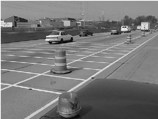
Rumble strip for work zone speed control
