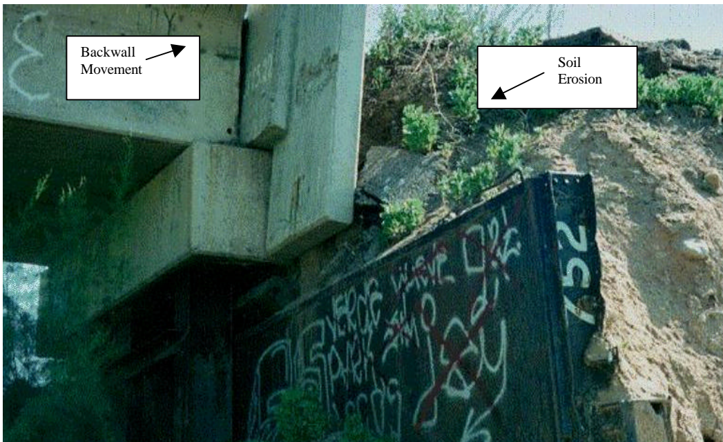
“Bridge MP 1195.22 - Backwall Movement Due To Erosion”
