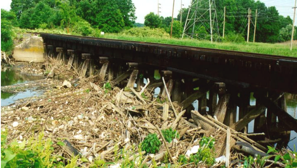
“Debris Buildup Next To Bridge”
