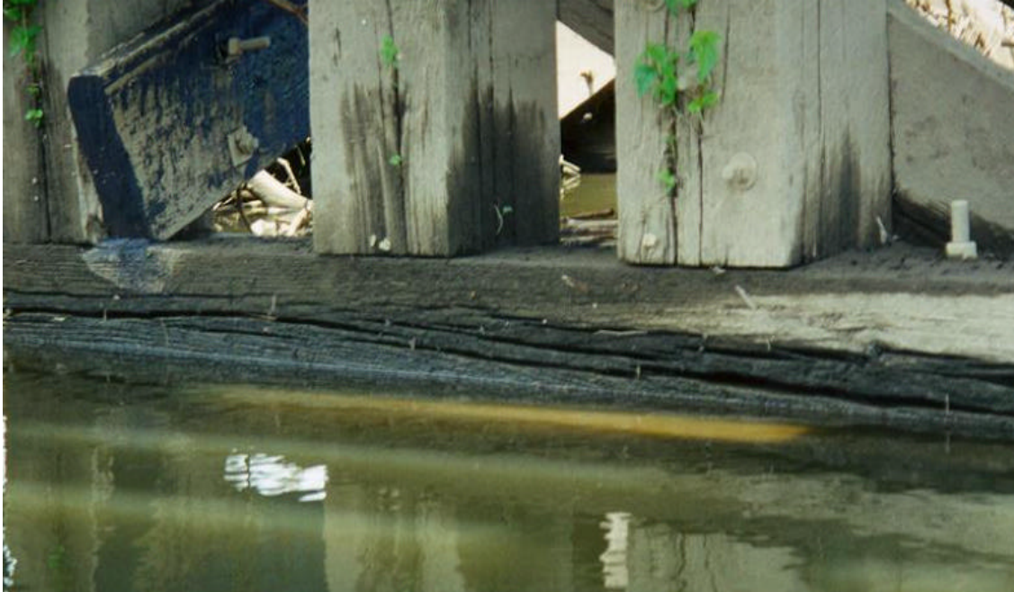
“Bridge 5.73 - Exposed Piers Subject To Decay”
