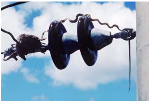
This snake died by electrocution as it crawled from the power pole across the insulator to the nest of a bird (drongo) situated on an active power line. A snake crossing an insulator can cause a power outage.
