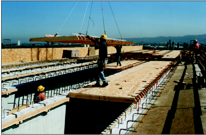
An agreement between Caltrans and the City of Oakland set goals for the employment of local residents, minorities, and women on the Cypress reconstruction project.
