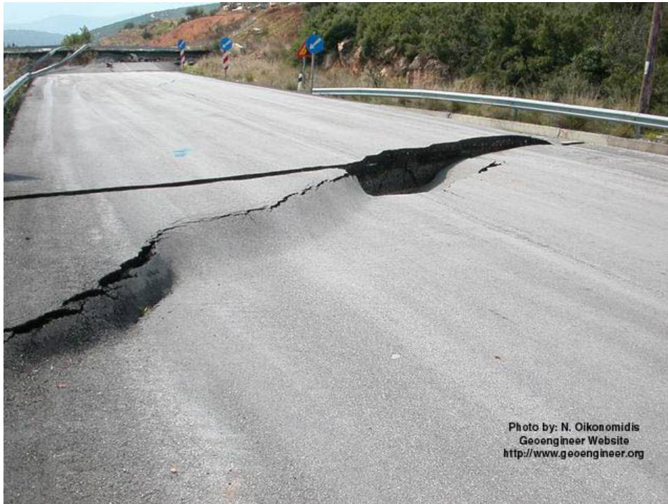
Figure 3-7. Slope failure beneath road pavement (www.geoengineer.com).
