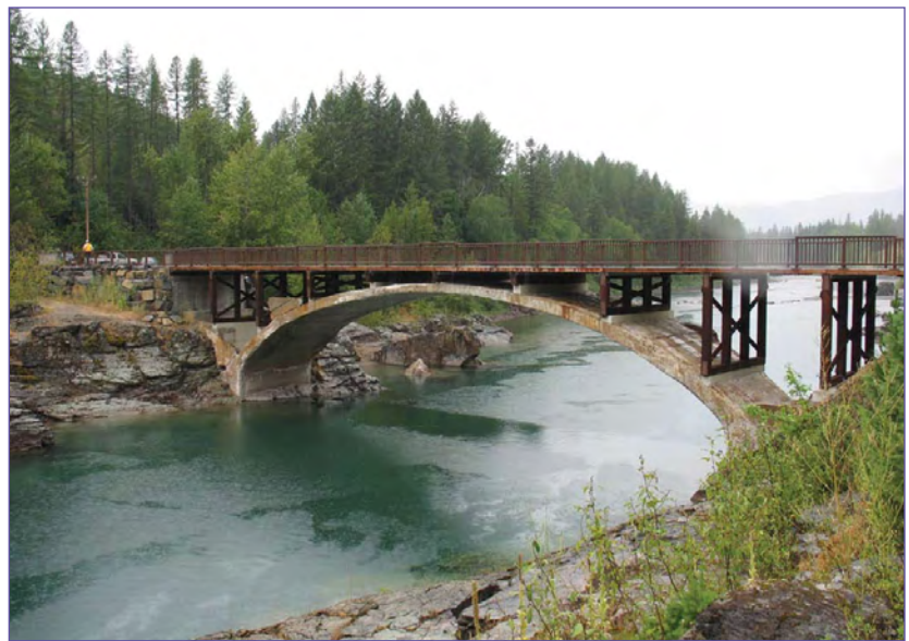
Belton Bridge across the Middle Fork of the Flathead River, Glacier National Park, Flathead County, Montana (National Park Service)
