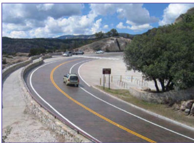
General Hitchcock Highway (Mt. Lemmon Highway, Arizona Forest Highway 39), Coronado National Forest, Tucson, Arizona (USDA Forest Service)
