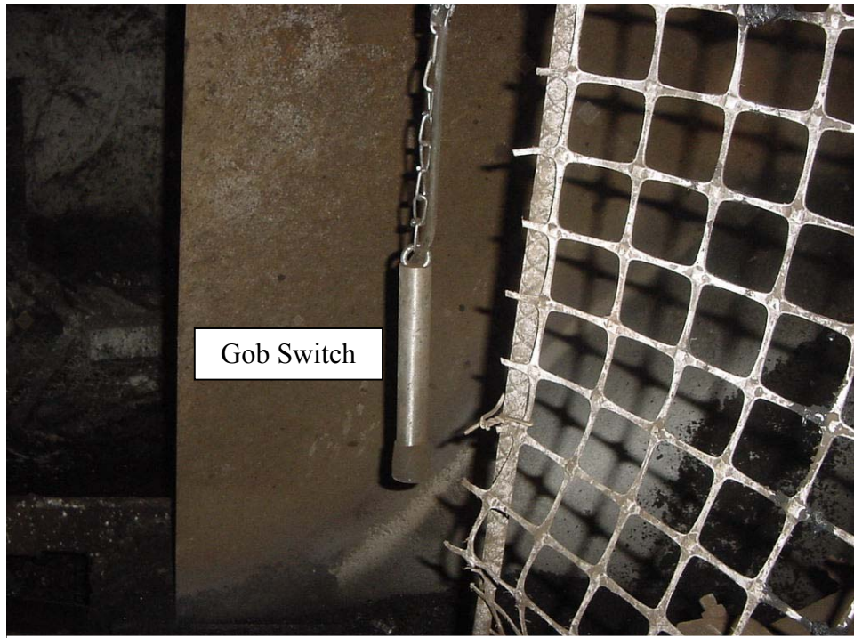
Figure #4 Gob Switch installed after the Fire
