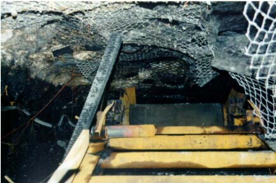
Figure #2 Fire Damage to the Top Area of the #2-3NW Belt
