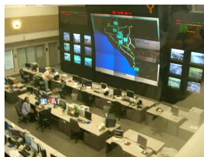
Caltrans District 12 TMC
