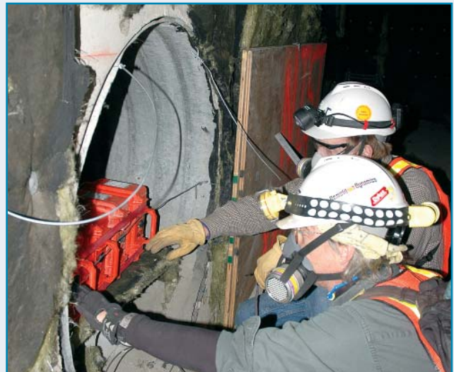
NIST electrical engineers Chris Holloway and Galen Koepke place transmitters in a protected air vent at the old Washington Convention Center prior to the implosion of the building. The experiments were performed to help improve the communication capabilities for emergency first responders.
