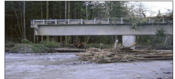
The damage to Boundary Bridge in 2003 will require a new bridge span.
