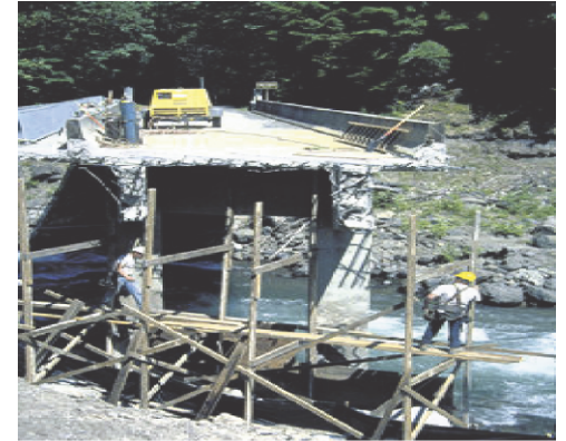
ERFO is funding repairs to this bridge over Iron Creek in Gifford Pinchot National Forest in Washington after it was devastated by a flood.
