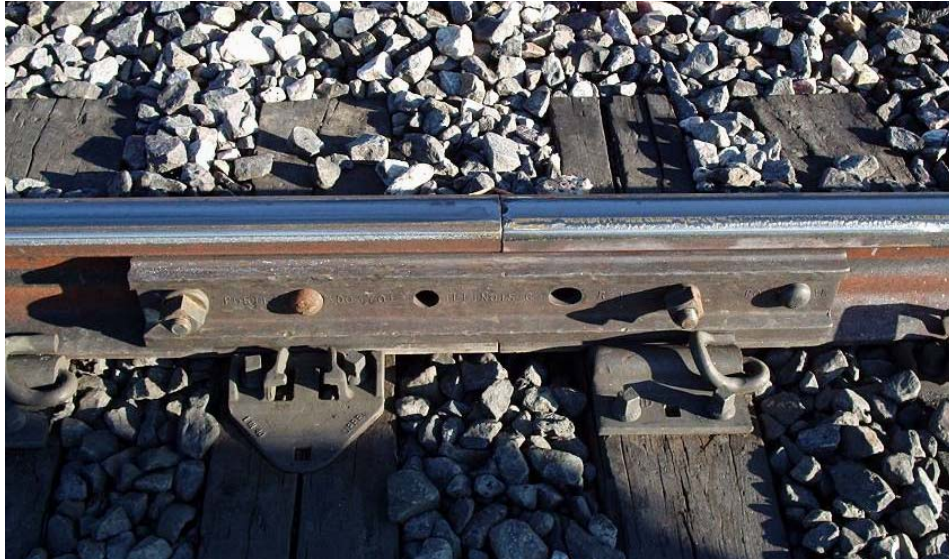
Figure 16. Junction of Control Rail to Laser-Treated Rail. Left Side is the Control Rail; Right Side is Laser-Treated Rail
