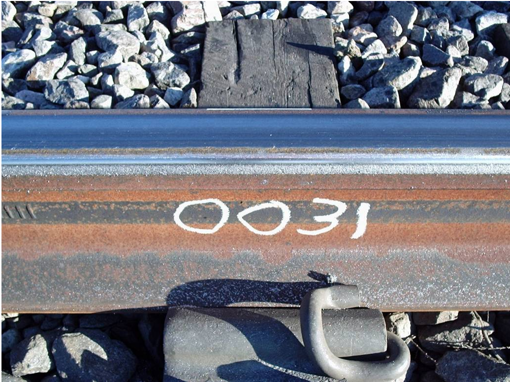
Figure 14. Control Rail Showing Rough Gage Face from Dry Operation. Shiny Gage Corner After 5.6 MGT
