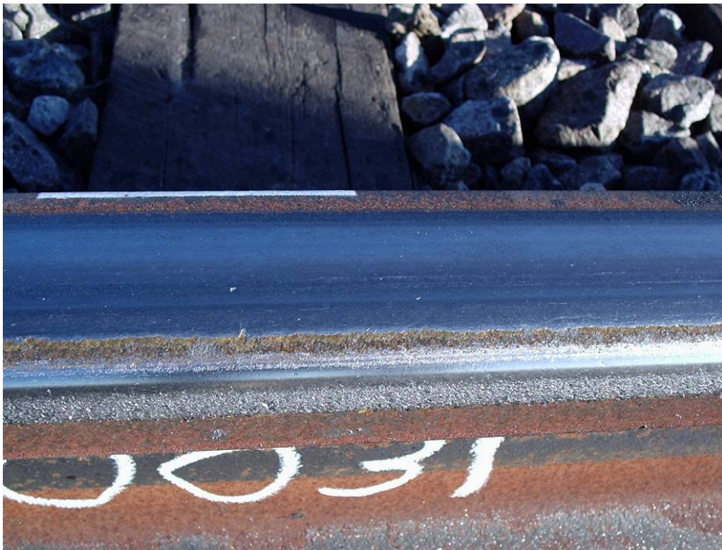
Figure 15. Control Rail Closeup Showing Dry Surfaces. No Pitting or Spalling After 5.6 MGT
