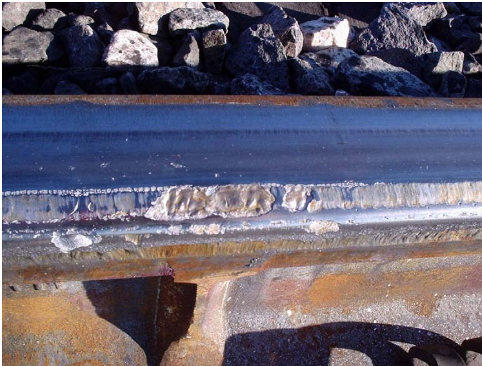
Figure 20. Close View of Spalls At and Near Thermite Weld After 5.6 MGT. Compare with Same Location as Shown in Figure 12 After 1.2 MGT
