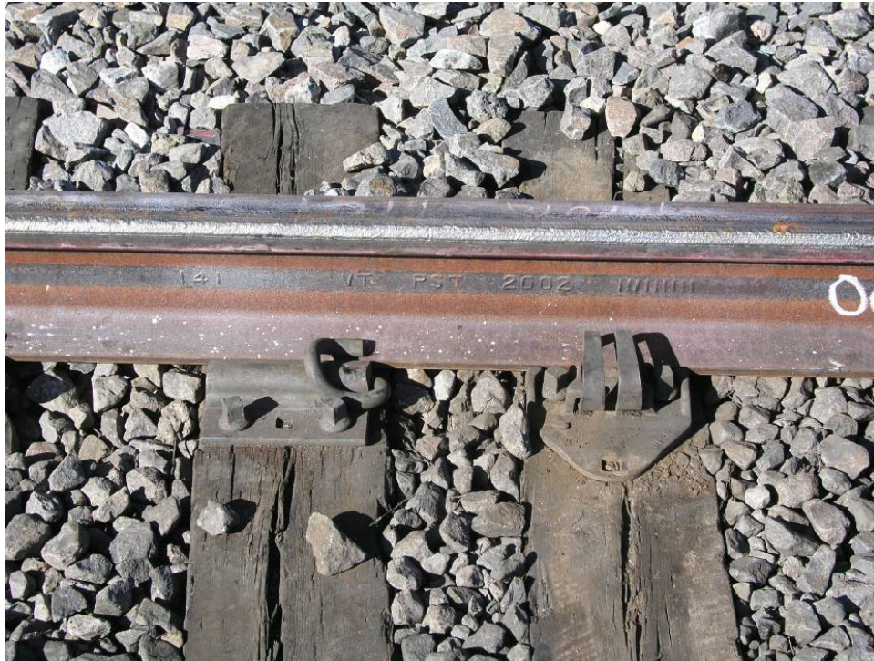
Figure 5. Laser-Treated Test Rail as Installed in Section 07 at FAST Before Train Operation
