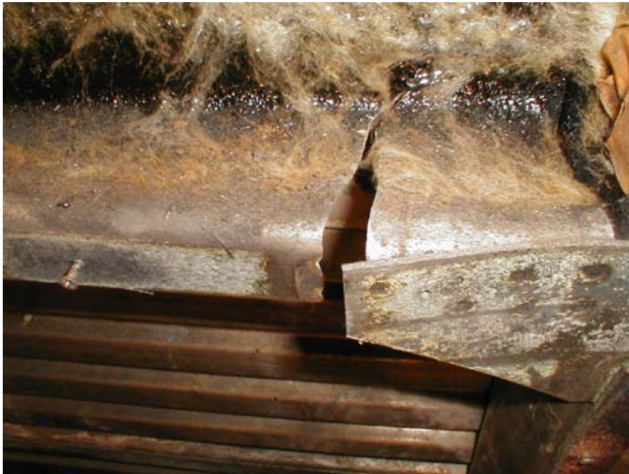
Figure B3-17. Right-side Belt Rail—Crack Detail Just Forward of Window Frame
