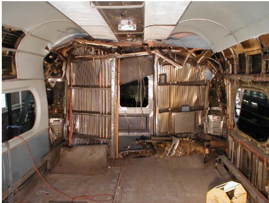
Figure 31. Internal View Looking Forward of Crushed End After Material Removal
