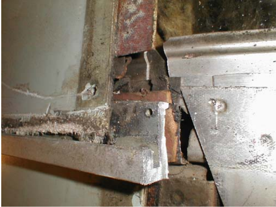
Figure B3-14. Left-side Cant Rail—Crack Detail Just Forward of Window Frame
