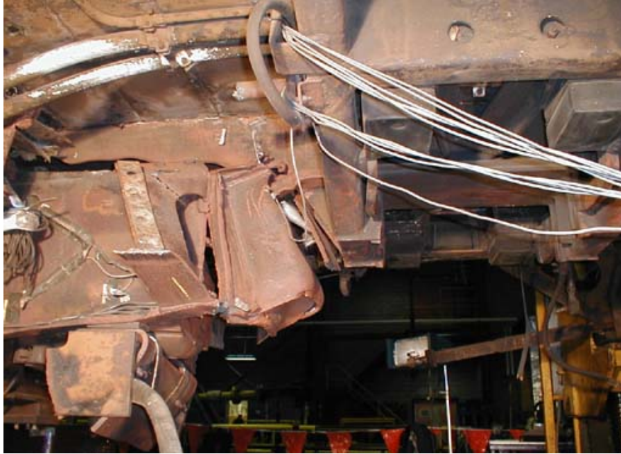
Figure B1-15. Aft Part of Draft Sill and Body Bolster Connection, from Left Looking Slightly Upward
