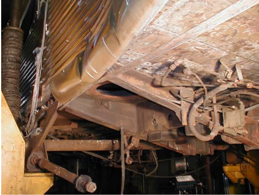
Figure B1-23. Right-side Bolster Beam Detail Showing Two Small Buckles, Forward Looking Aft
