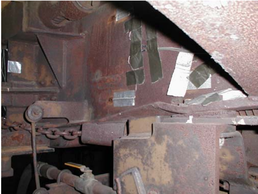
Figure B5-2. Aft Draft Sill - Buckle of the Draft Sill Flange Above Pilot Connection Plate
