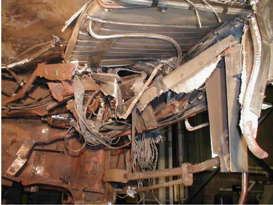
Figure B1-21. Right-side Forward Draft Sill and Underside of Floor Prior to Removing Trap Door
