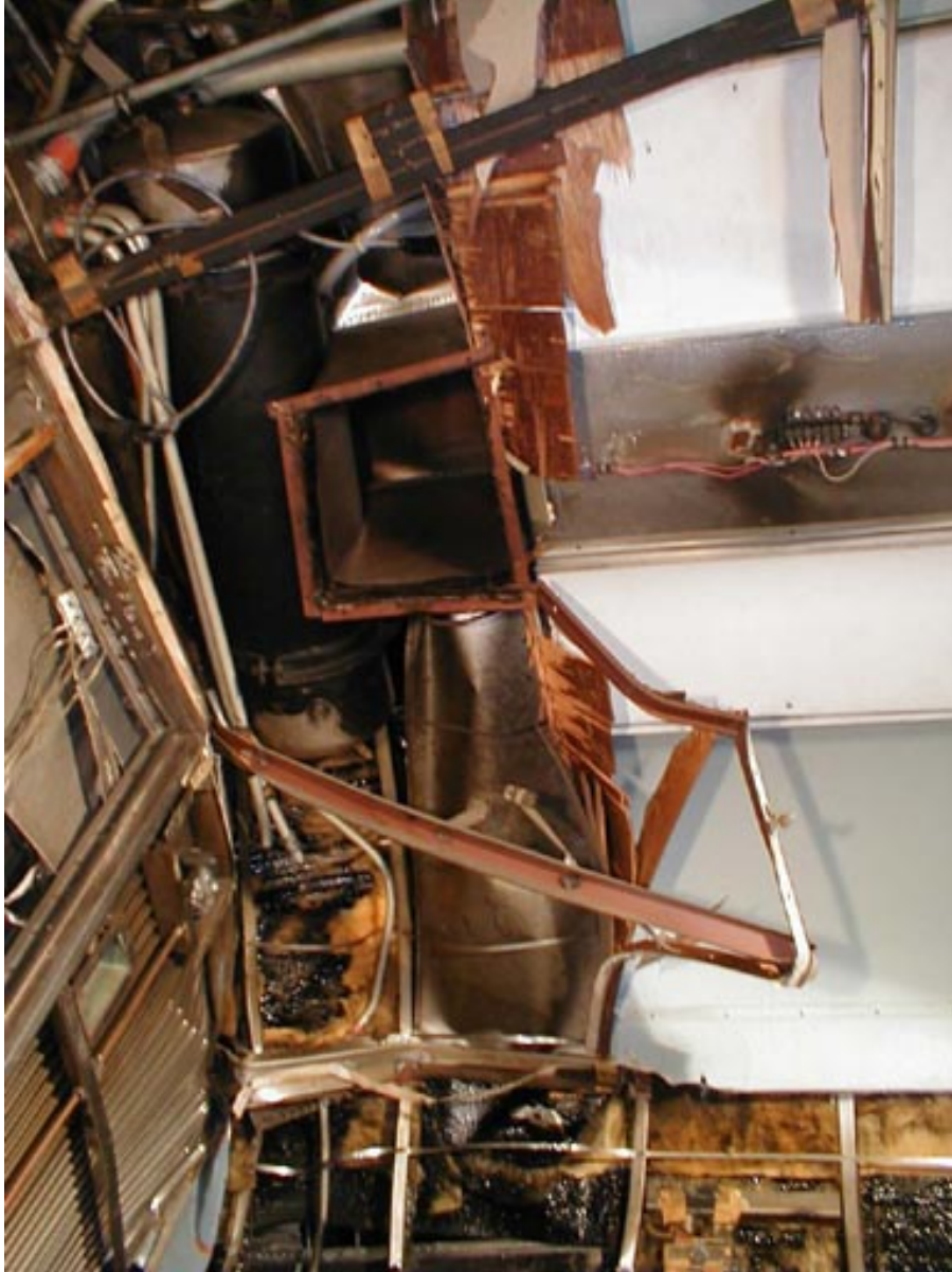
Figure B3-24. Ceiling Damage Aft of Bulkhead Wall—View from Below
