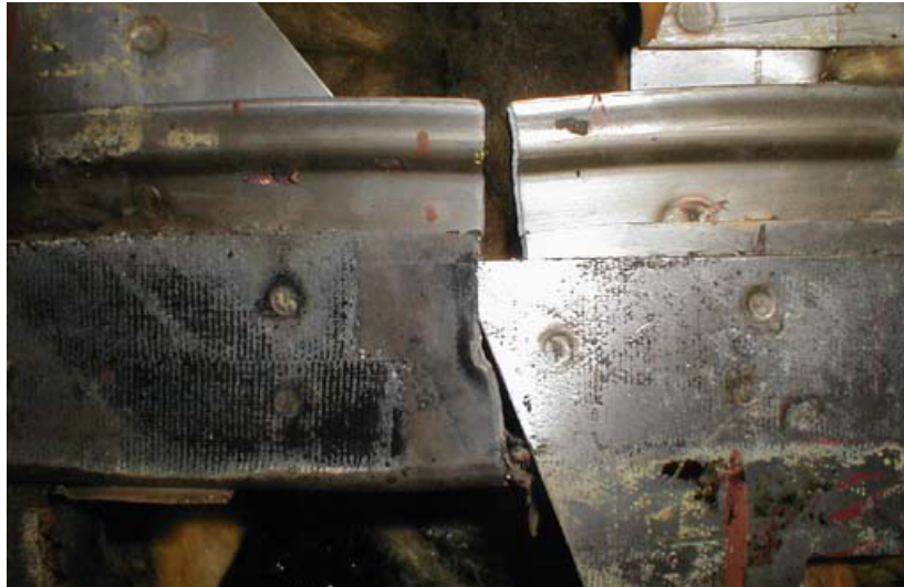
Figure 22. Right-side Cant Rail—Crack Detail Just Forward of Window Frame
