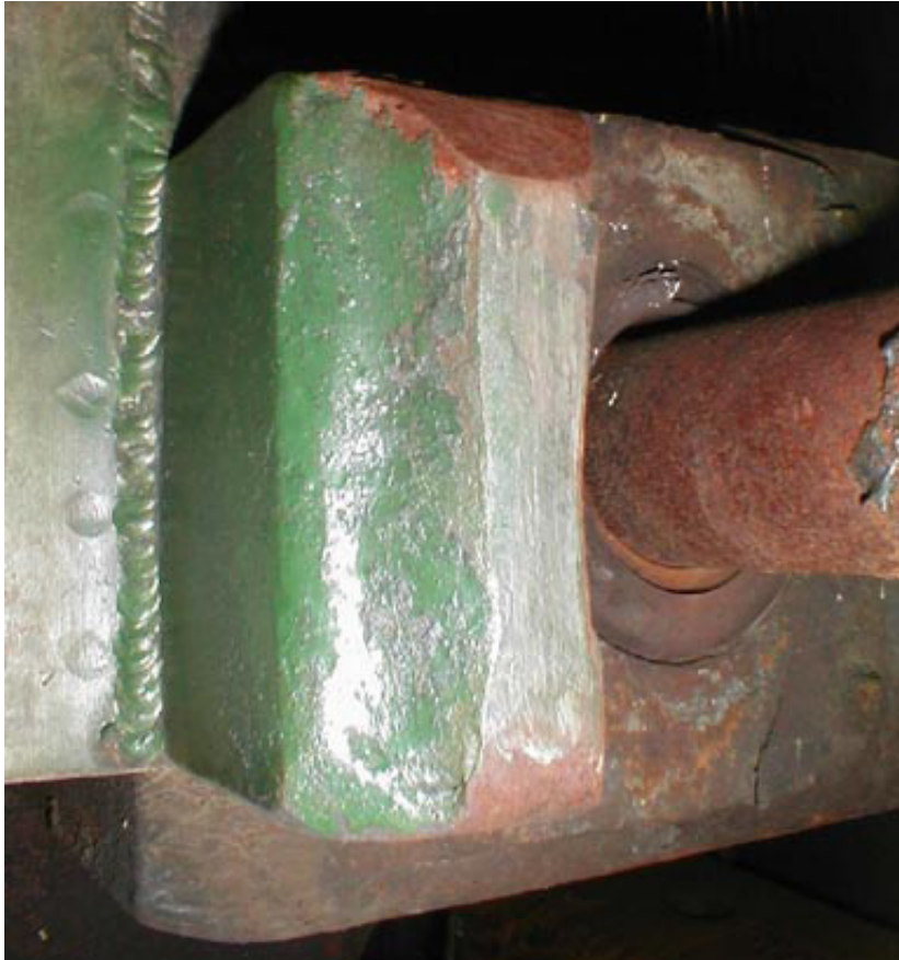
Figure B5-11. B-End Buff Stop—Collision Marks from Impact with Trailing Car
