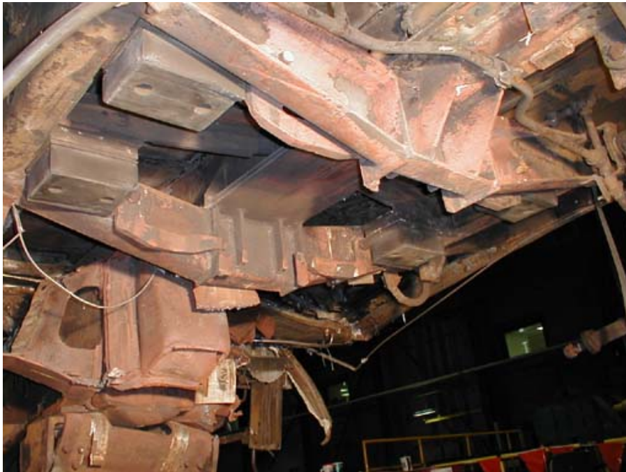
Figure B1-18. Detail of Body Bolster Without Bolster Beam. Aft Looking Forward from Left Side
