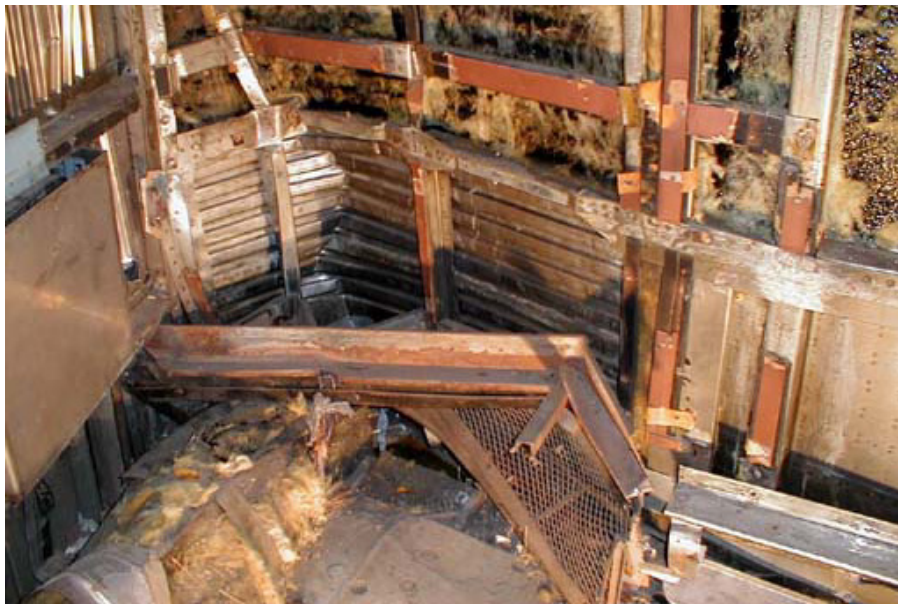
Figure B3-12. Composite Showing Forward Right-side Wall Between Bulkhead Wall and First Window Frame
