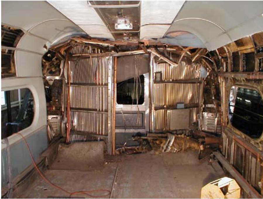
Figure B3-20. Internal View Looking Forward of Crushed End After Material Removal
