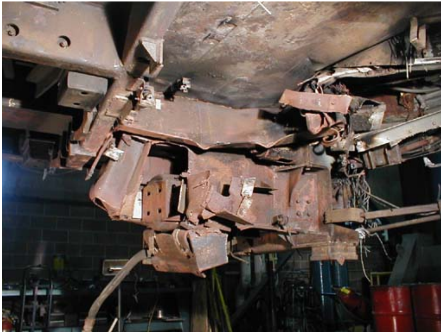
Figure B1-26. Draft Sill - Right-side Deformations
