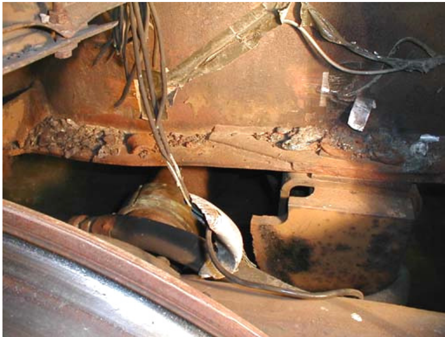
Figure B1-8. Draft Sill Collapse Detail with Truck Attached, From Left Side (note pilot attachment hardware aft and below center line of front axle)
