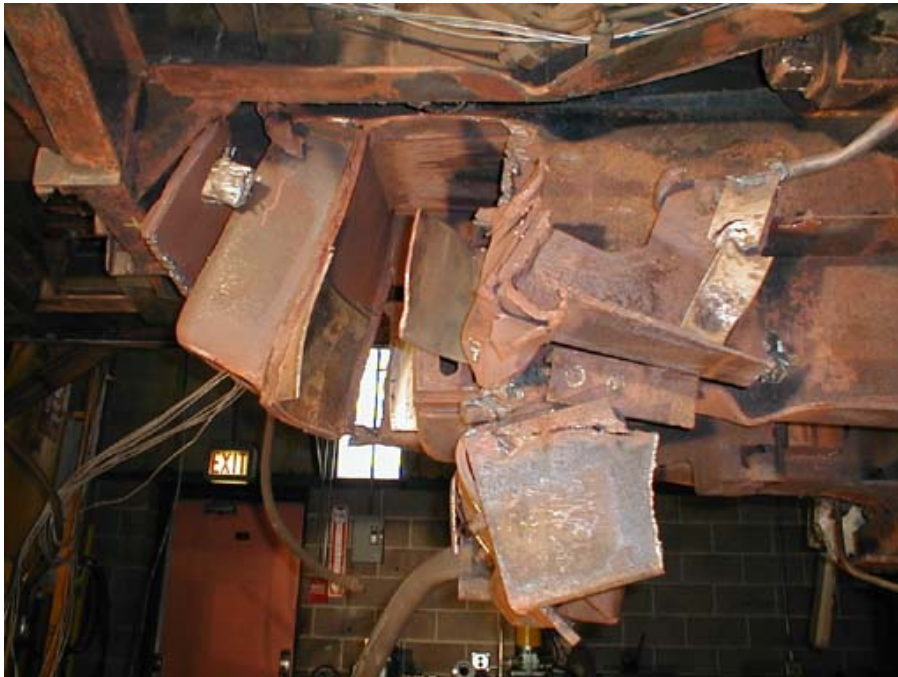
Figure B1-12. Aft Part of Draft Sill and Body Bolster Connection, from Right Looking Slightly Upward
