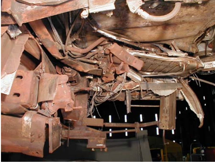
Figure B1-19. Right-side Draft Sill Collapse and Forward Underframe Before Removing Trap Door, Aft Looking Forward
