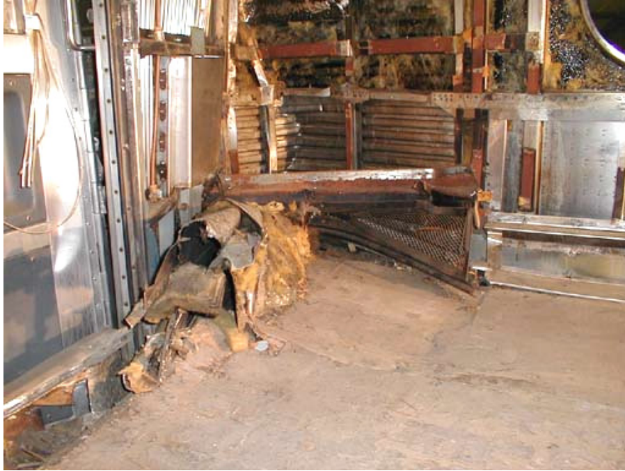
Figure B3-18. Right-side Floor Buckling and Seat Frame Aft of Bulkhead Wall
