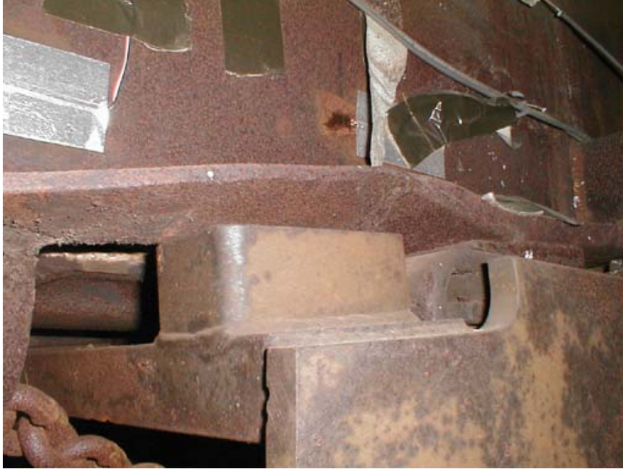
Figure B5-3. Aft Draft Sill - Buckle of the Draft Sill Flange Above Pilot Connection Plate
