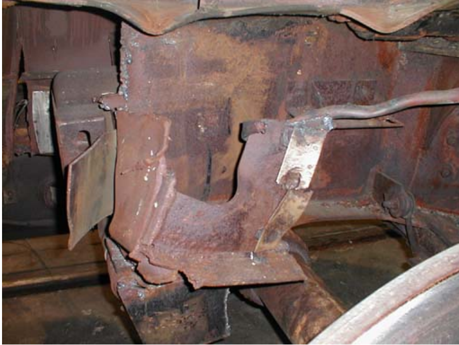
Figure B1-7. Draft Sill Collapse Detail with Truck Attached, From Right Side (note pilot attachment hardware aft and below center line of front axle)
