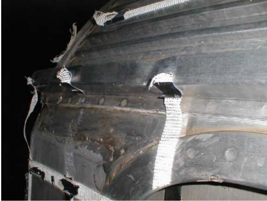
Figure B5-7. Buckle in Rain Gutter Above Top Left Corner of Right-Rear Door Frame
