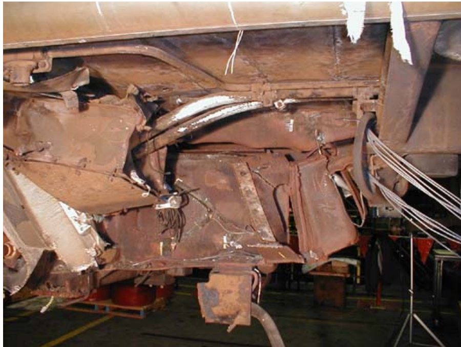
Figure B1-16. Left-side Draft Sill Between Body Bolster and Vestibule Wall Bolster
