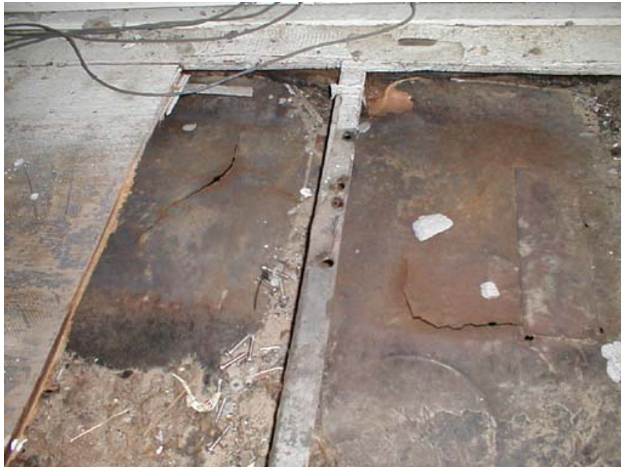
Figure B3-8. Cracks in Floor Sheathing Under Removed Floor Panels
