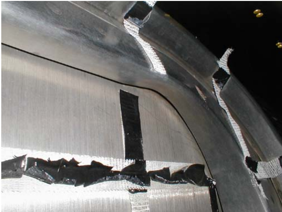
Figure B5-8. Buckle in Top Right Corner of Right-Rear Door Frame – Outside
