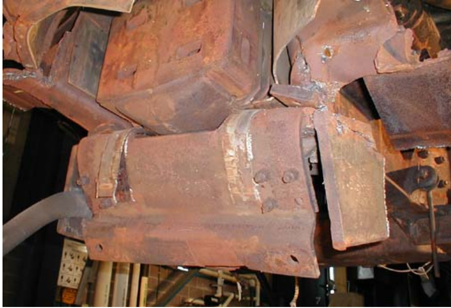
Figure B1-31. Forward Draft Sill Detail - Deformation of Pilot Connection Plate Under the Draft Gear
