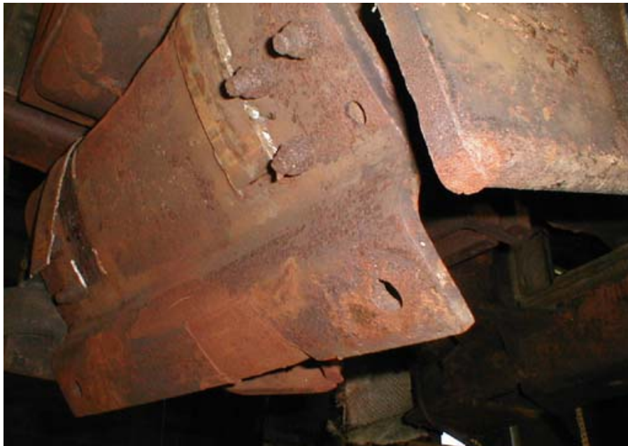
Figure B1-32. Forward Draft Sill Detail Showing Effects of Impact with the Front Axle
