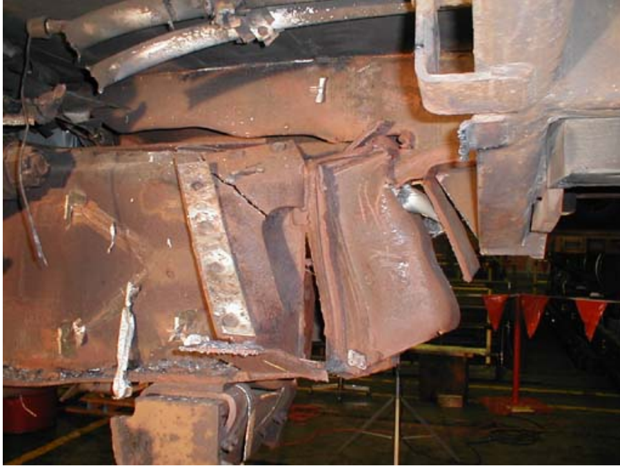
Figure B1-25. Left Side of Draft Sill - Impact of Buff Stop Against Body Bolster
