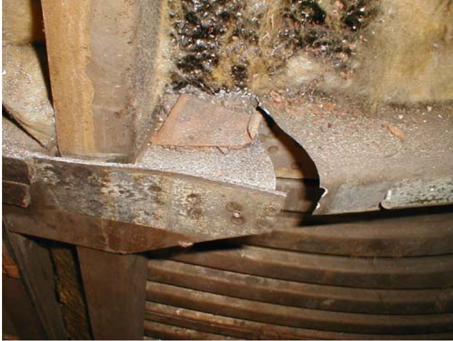
Figure B3-16. Left-side Belt Rail—Crack Detail Just Forward of Window Frame
