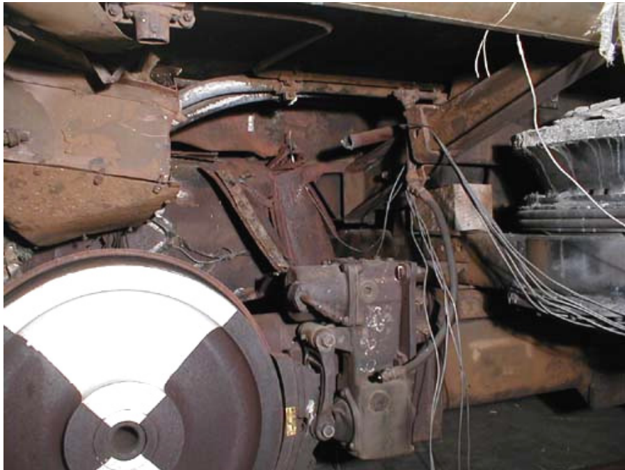
Figure B1-4. Left-side Draft Sill Collapse Before Truck Removal
