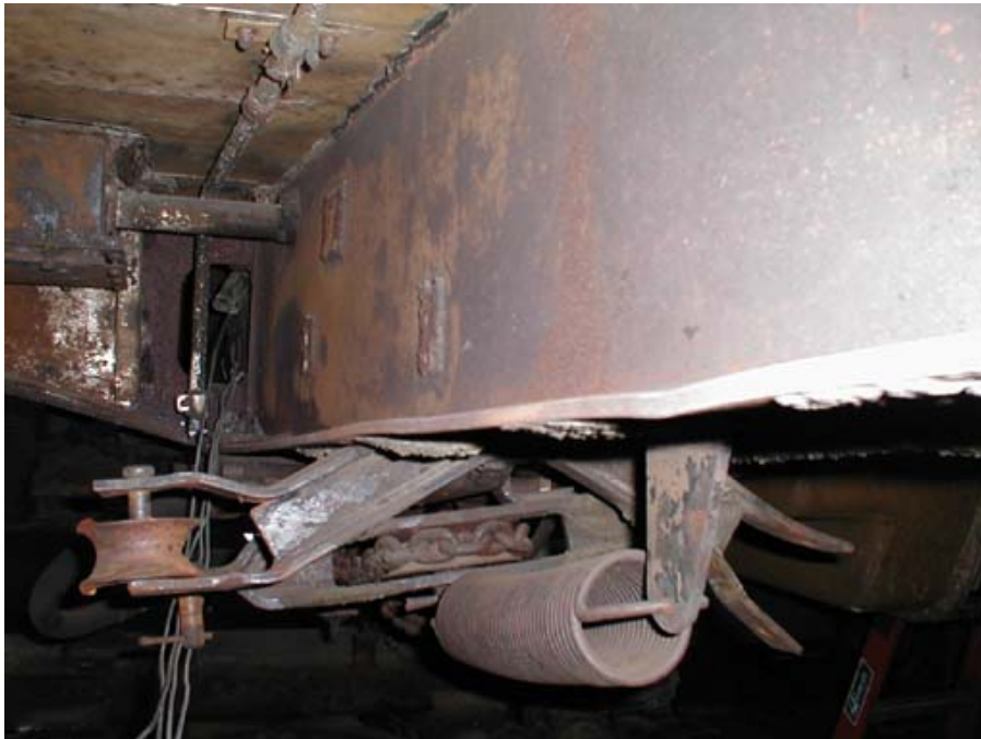
Figure B5-4. Aft Draft Sill - Slight Buckling of the Draft Sill Flange
