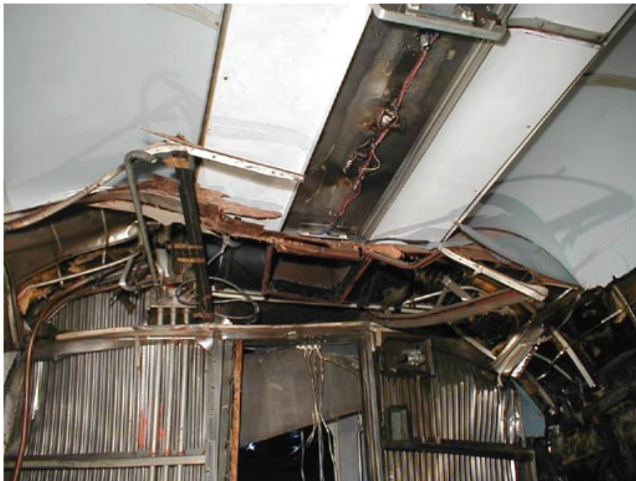
Figure B3-21. Upper Damage aft of Bulkhead Wall—View After Material Removal
