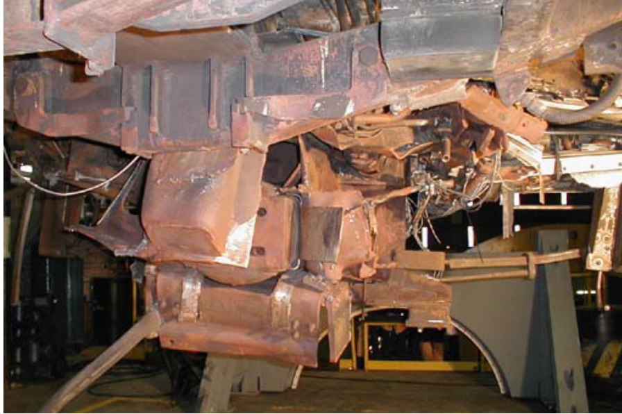
Figure B1-13. Draft Sill Collapse from Behind, Slightly on Right Side, Aft Looking Forward
