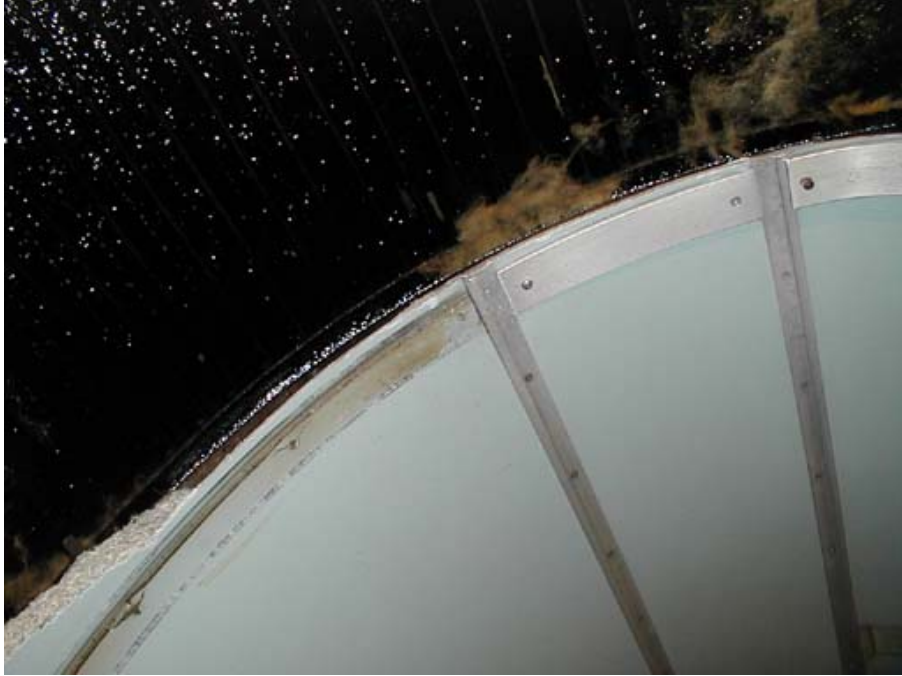
Figure B3-9. Coating in Inside Surface of Upper Sheathing in the Carbody
