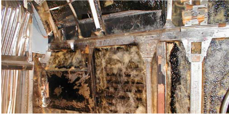
Figure 21. Right-side Cant Rail Between Window Frame (right) and Bulkhead Wall (left)
