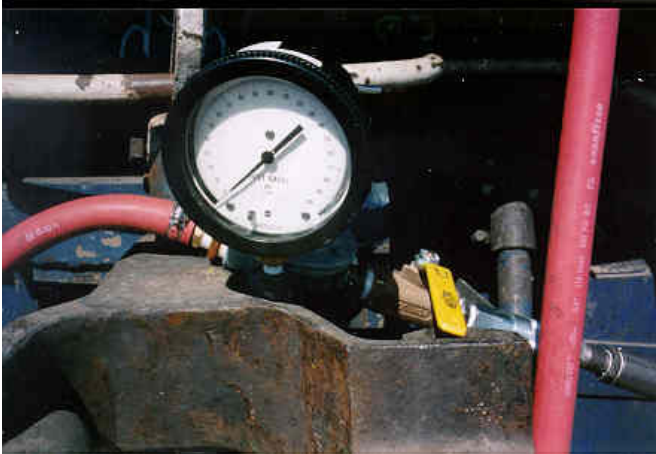
Figure 9. Air Pressure Control Valve/Pressure Gauge
