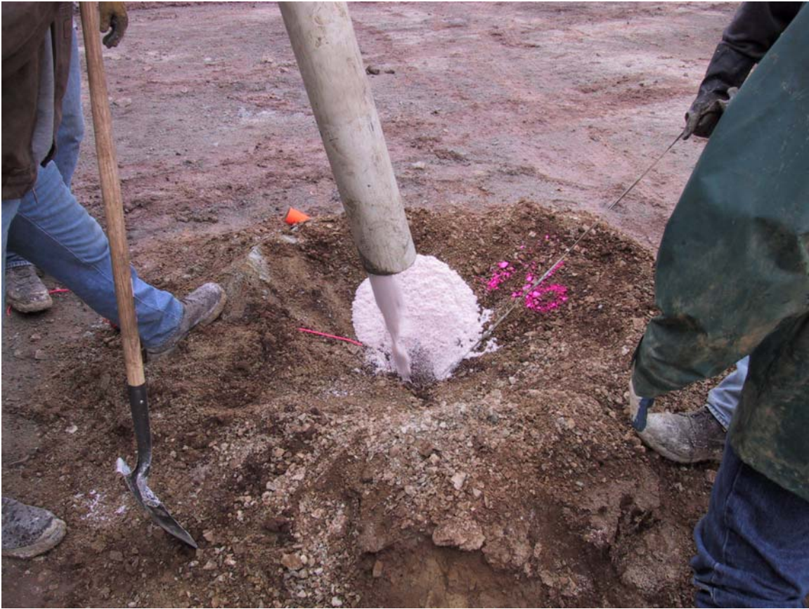
Figure 9 - Loading ANFO into a blast hole primed with a booster and Daveytronic® electronic
