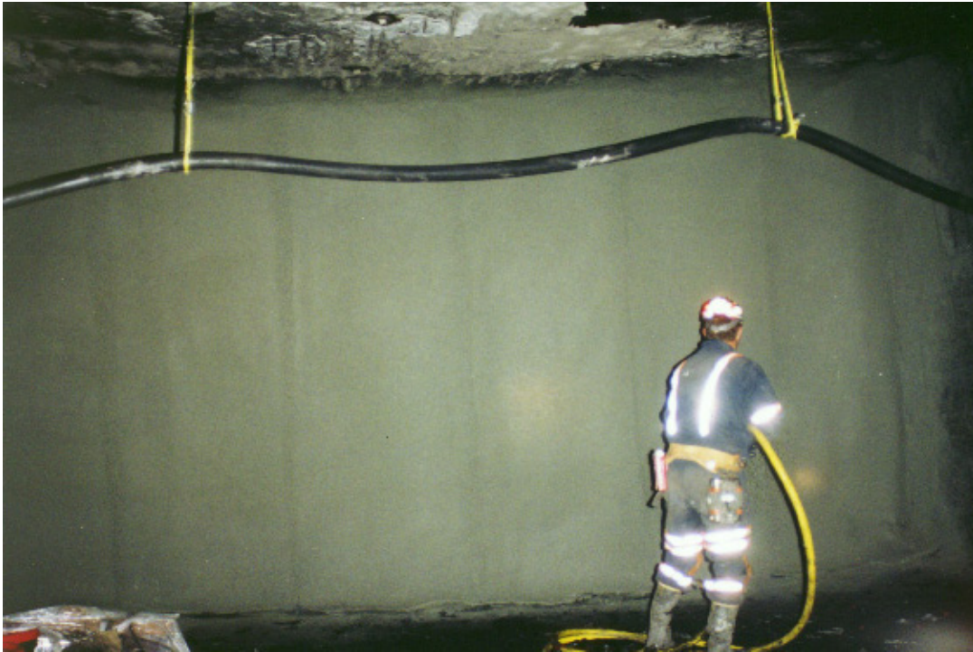
Figure 3 - A “Nontraditional” Stopping Constructed and being Sprayed with Cementitious Material in a Coal Mine
