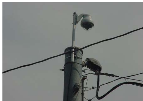
Figure 6-55 Portable CCTV Camera Mounted on Traffic Signal Pole (6)
