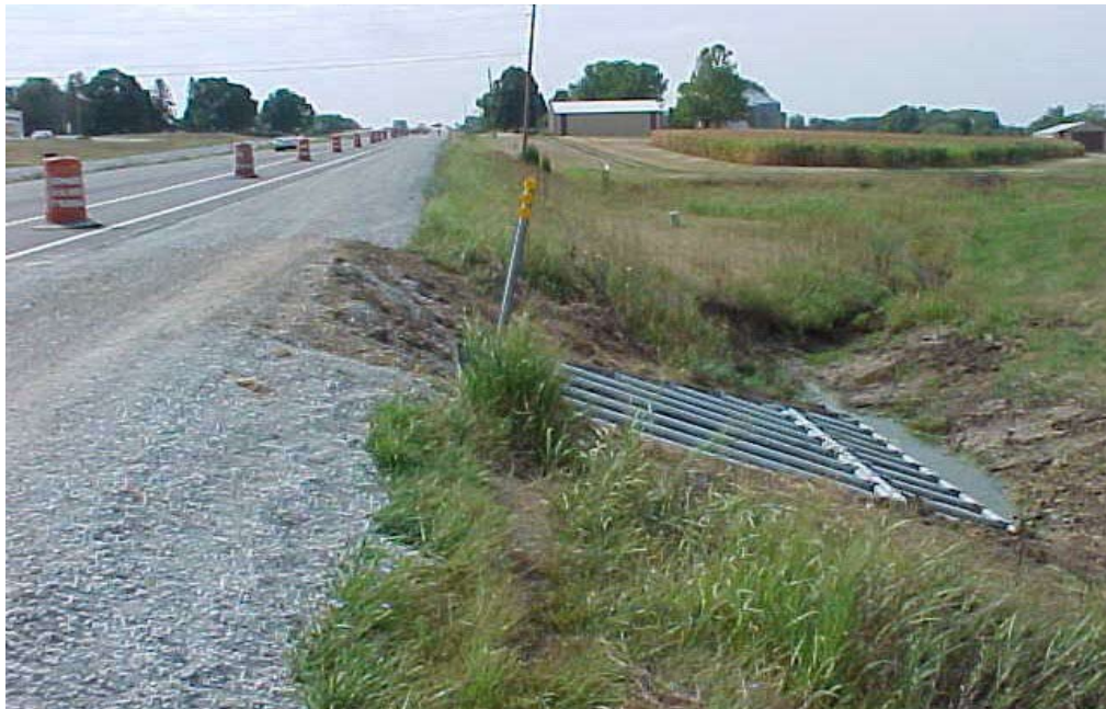
Figure 17. Traversable culvert grate, Iowa. (Source: Courtesy of IADOT)
