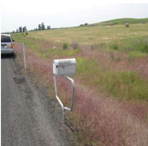
Figure 23. Crashworthy mailbox installation in Washington State.
