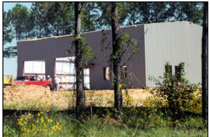
Construction of the new Southeast Regional Training Facility and home to the Jackson Hotshots will be completed early in 2004.
