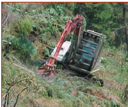
The contractor is shown piling the slash with the use of an excavator.
