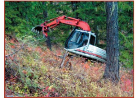
The eight ton excavator with rake attachment and boom reach of 25 feet helped in thinning.
