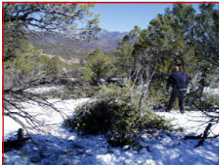
Taos Pueblo crew members working on BLM's Cooper Hill wildland-urban interface project.
