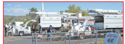
The combination chipper hauler trucks from Arizona Public Service were a huge help on the project, clearing large piles of brush in a matter of minutes.
