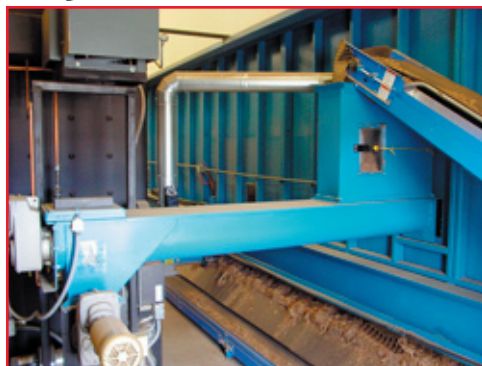
A conveyer belt moves wood chips from the storage bin on the right to the furnace, shown on the left.
