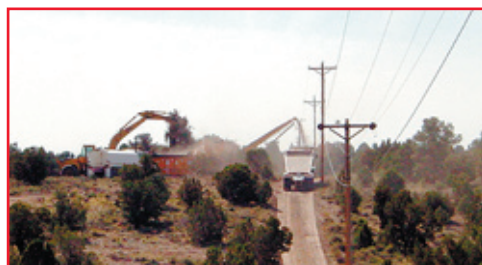
The BLM contractor uses an excavator to feed felled pinyon-juniper to the shredder. Biomass is subsequently loaded into the waiting semi-truck.
