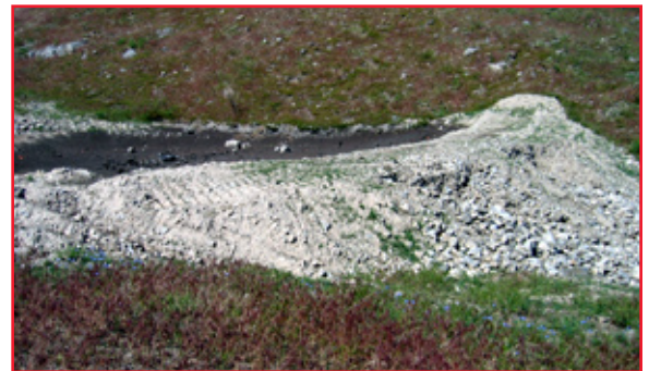
The spring of 2005 represented one of the wettest seasons on record, with record flows of runoff in the area. This catch basin represents many that were filled to overflowing capacity, going over the top. Like many, this catch basin was damaged but it did its job of slowing sediment and runoff flow in a highly above normal water year. It is planned that these sediment catch basins will be repaired and cleaned out this fall.
