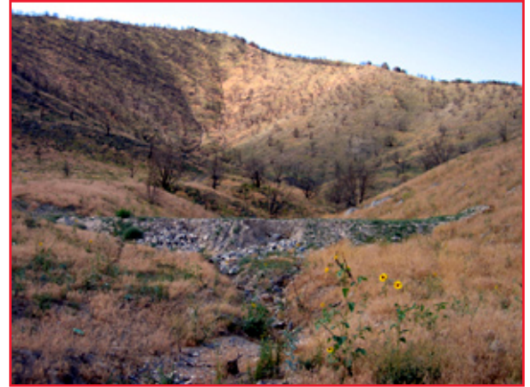
Typical sediment catch basin on the Concrete stabilization project. Runoff sediment was caught to prevent flood runoff onto private and public land. At least 70 of these structures aided in slowing the flow of water and mud.
