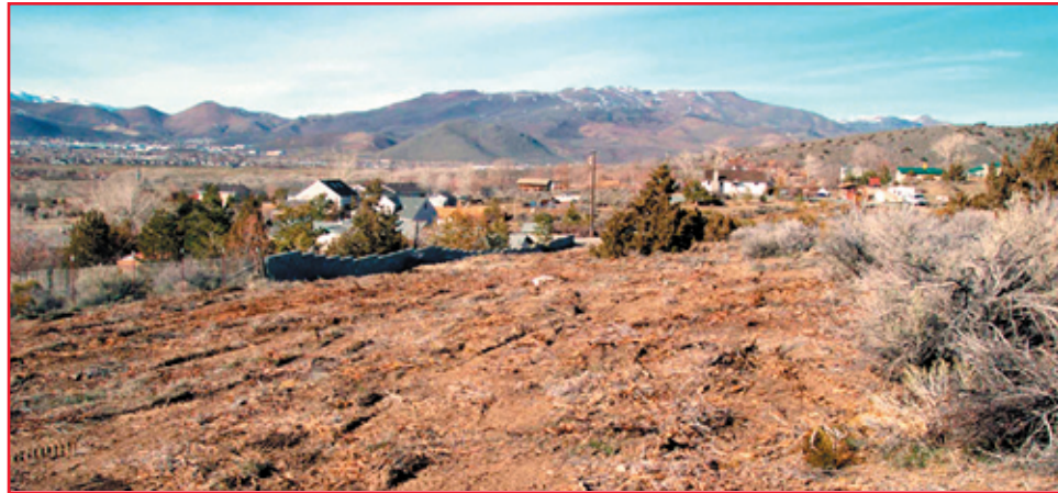
Joe Fording of the Nevada Division of Forestry supervises crews thinning flammable fuels and creating defensible space on private property.
