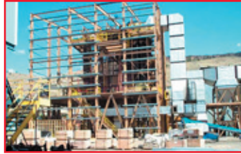
Cogeneration facility at the Confederated Tribes of the Warm Springs reservation in central Oregon.
