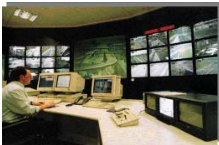
Figure 53. CITRAC and NADICS traffic management center, Glasgow.
