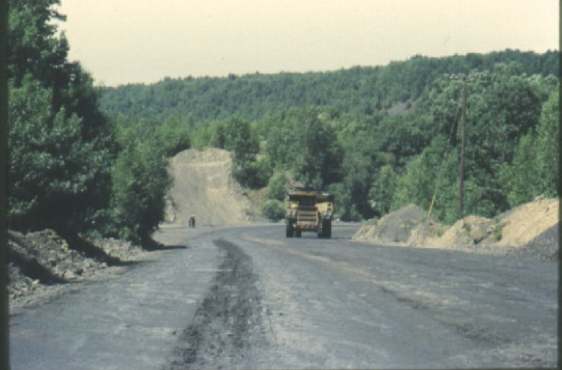
Here's an example of an escape ramp. The ramp is still under construction in this picture, but in the first year after it was completed, a runaway truck was saved on the ramp.
