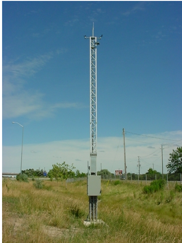
Figure 15-12: Environmental Sensor Station
