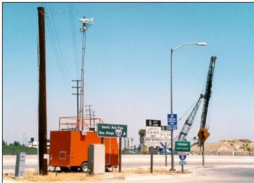
Figure 15-11: Portable CCTV Assembly
