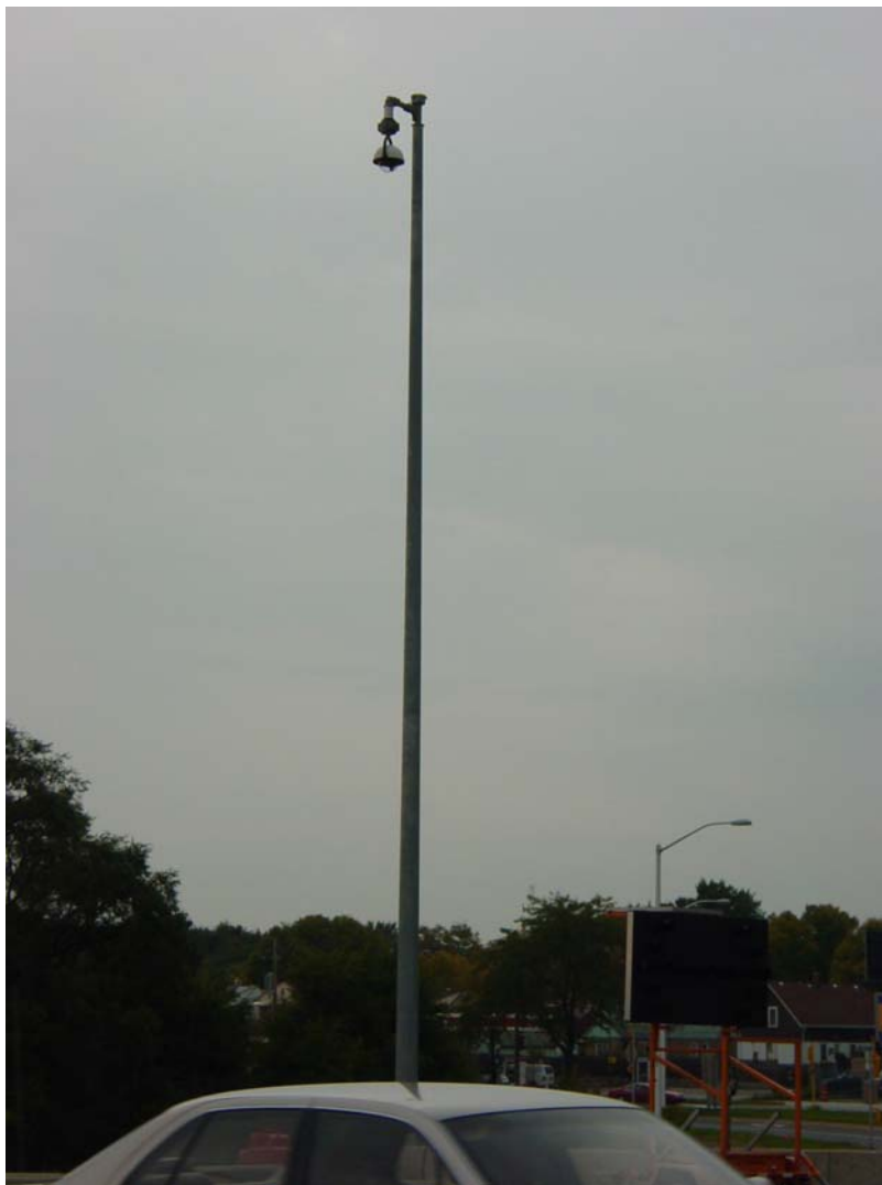
Figure 15-10: CCTV Camera Assembly
