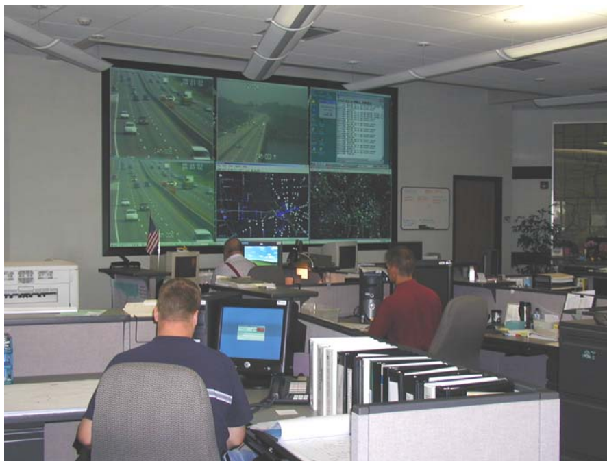
Figure 14-1: Transportation Management Center
