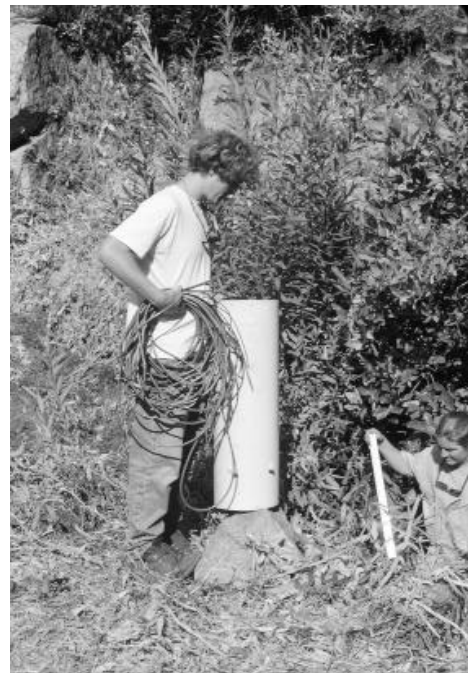
Figure 12. Installing stilling well to house a pressure transducer and thermistors to collect stream height and temperature data at the road culvert over Trauger's Creek.
